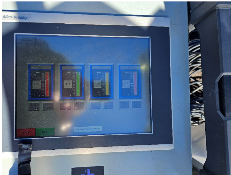
Figure 13: HMI Readout: Post-Operation Final Readings
