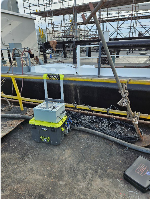
Figure 11: HMI and Cables on wing wall
