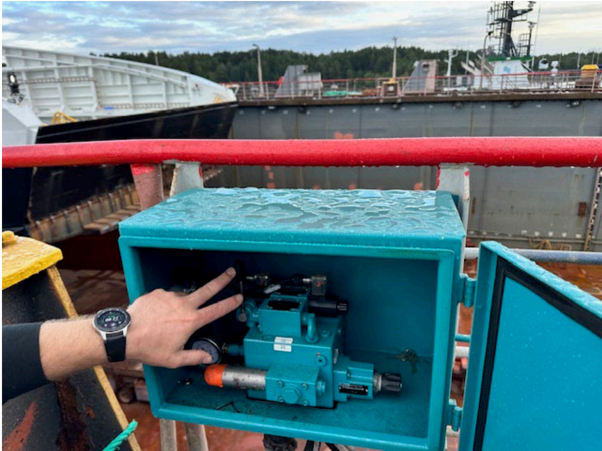
Figure 6: Photo of Bilge Support Arms Local Controls
