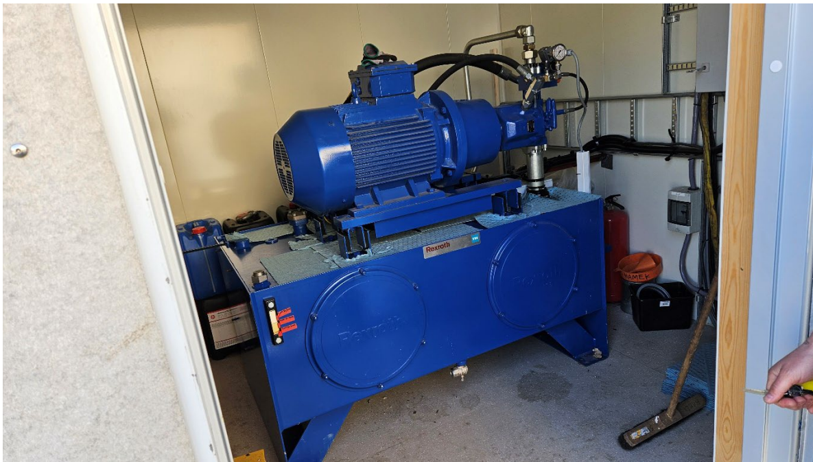
Figure 11: Photo of Sidewall Support HPU
