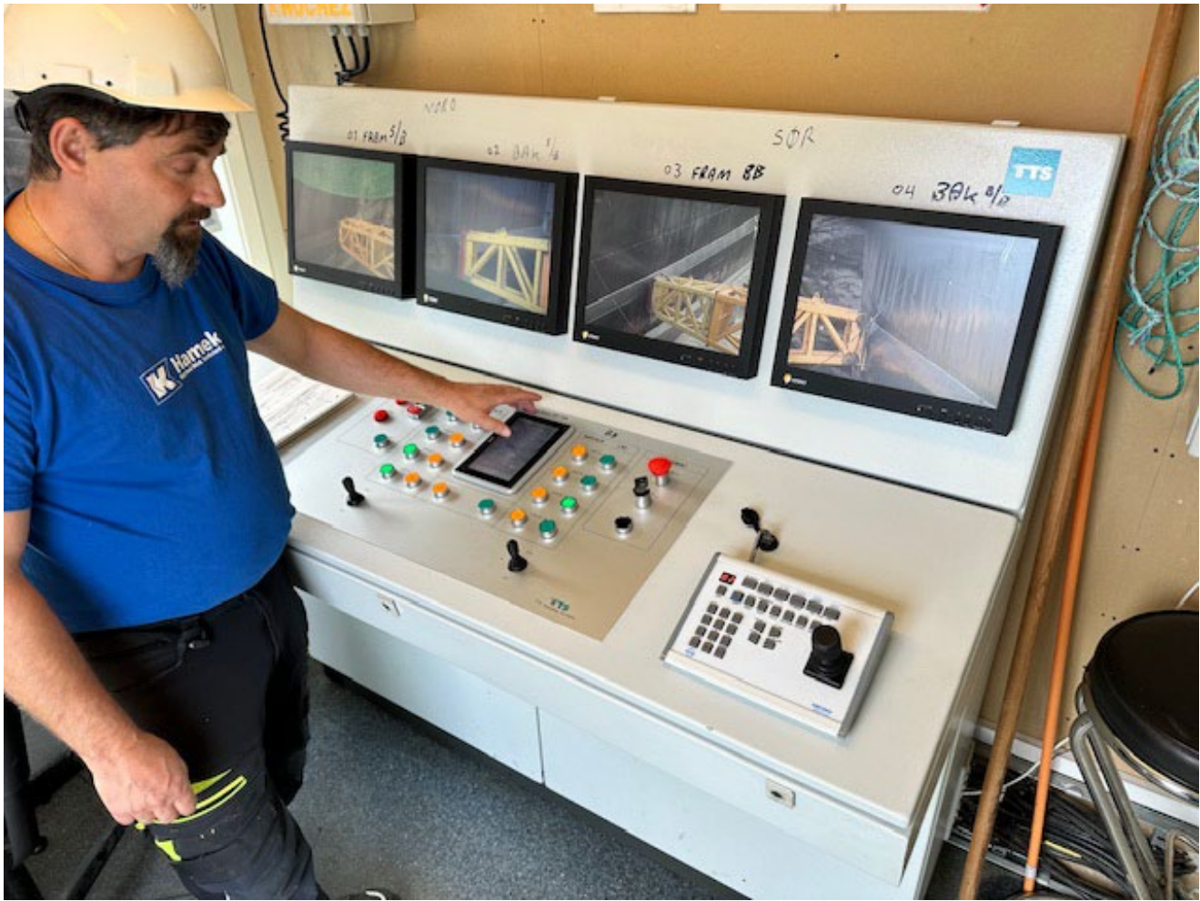
Figure 12: Photo of Sidewall Support Control Console
